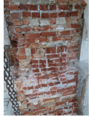
freeze-thaw brick backup masonry
