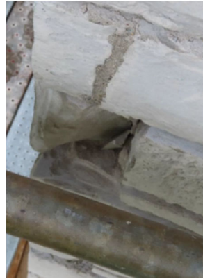
spalled lannon stone
