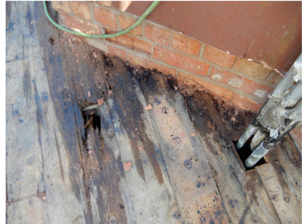
rotted decking — part of cricket
