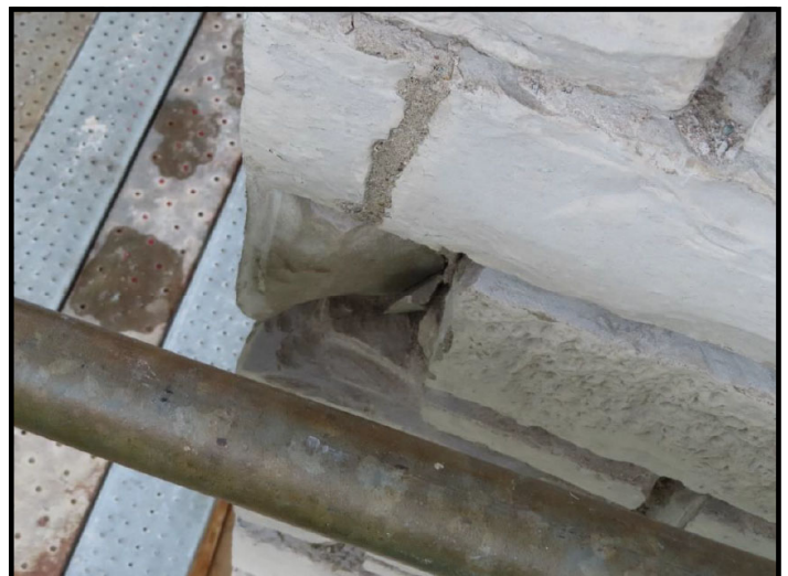
A spall observed from the scaffold.
