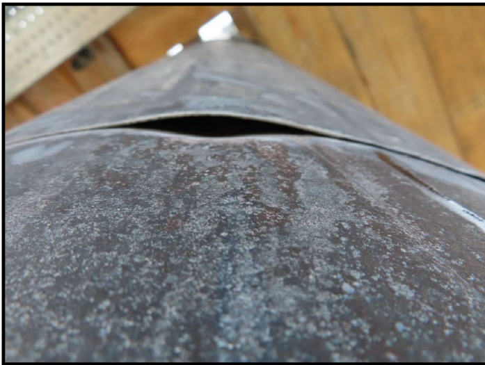
A gap in the lead coated copper cladding.
