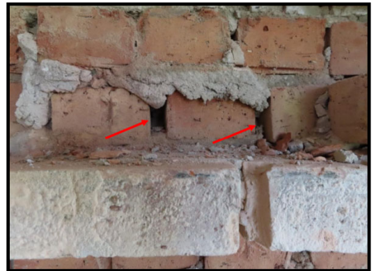
Voids present in the backup masonry of the belfry.
