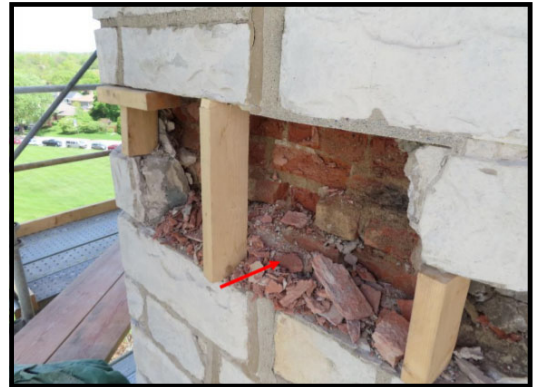
The inspection opening below spire on the west elevation. Note the delaminated brick exhibiting freeze-thaw damage.
