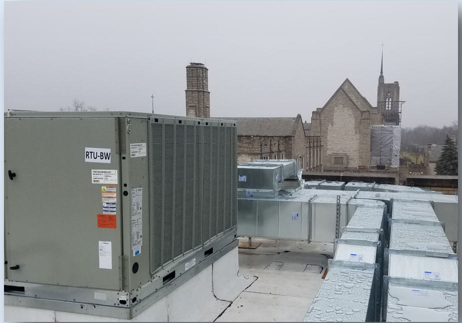
Rooftop Air-Conditioning Unit
