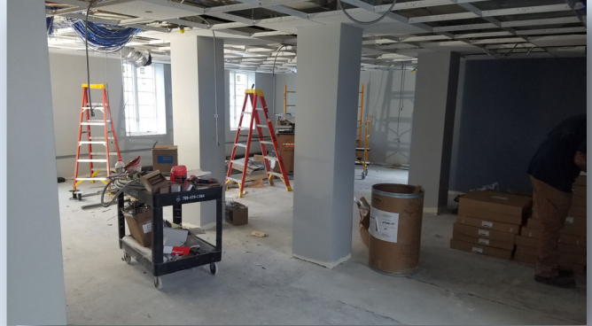
3rd Floor SPREAD Room
